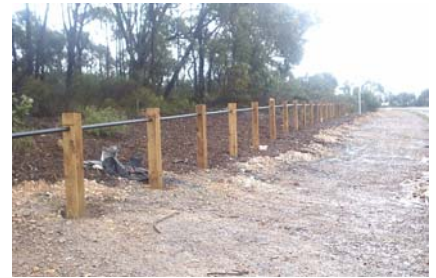
Above, Permanent fence around endangered ecological community promised by February, still not complete today.
